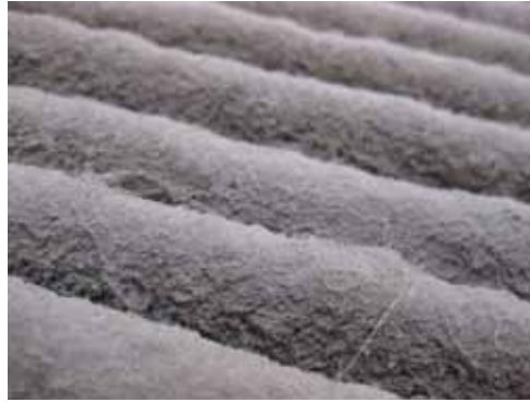
Air filters trap a lot of debris that otherwise would end up back in the house, stuck in ductwork, clogging HVAC equipment, or in our lungs.
